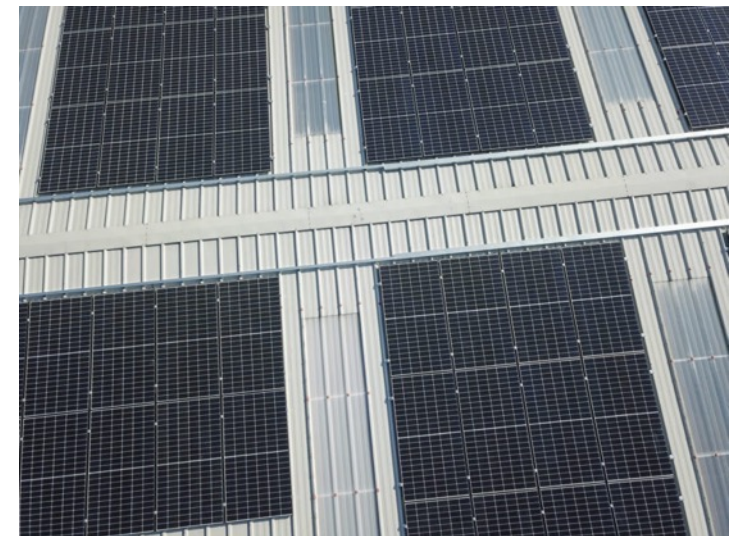
Astatine 120KW Wicklow Wolf Installation
